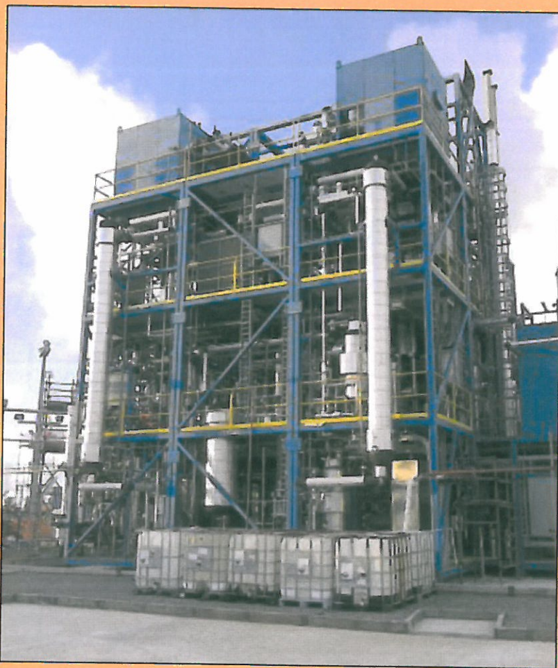
Development: the CompactGTL small-scale GTL facility
